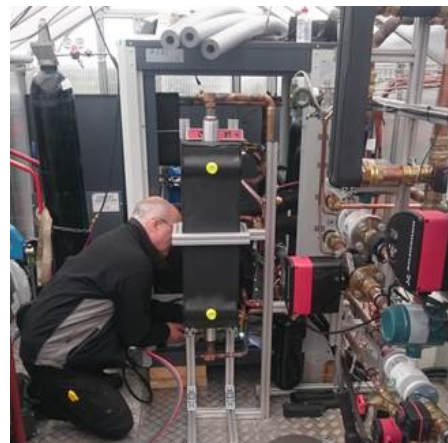
Condenser in preparation for testing
